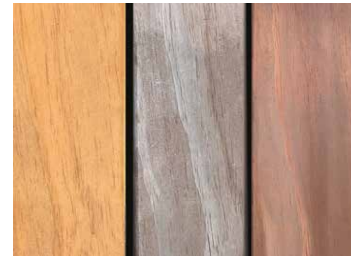
Ticari newly installed
